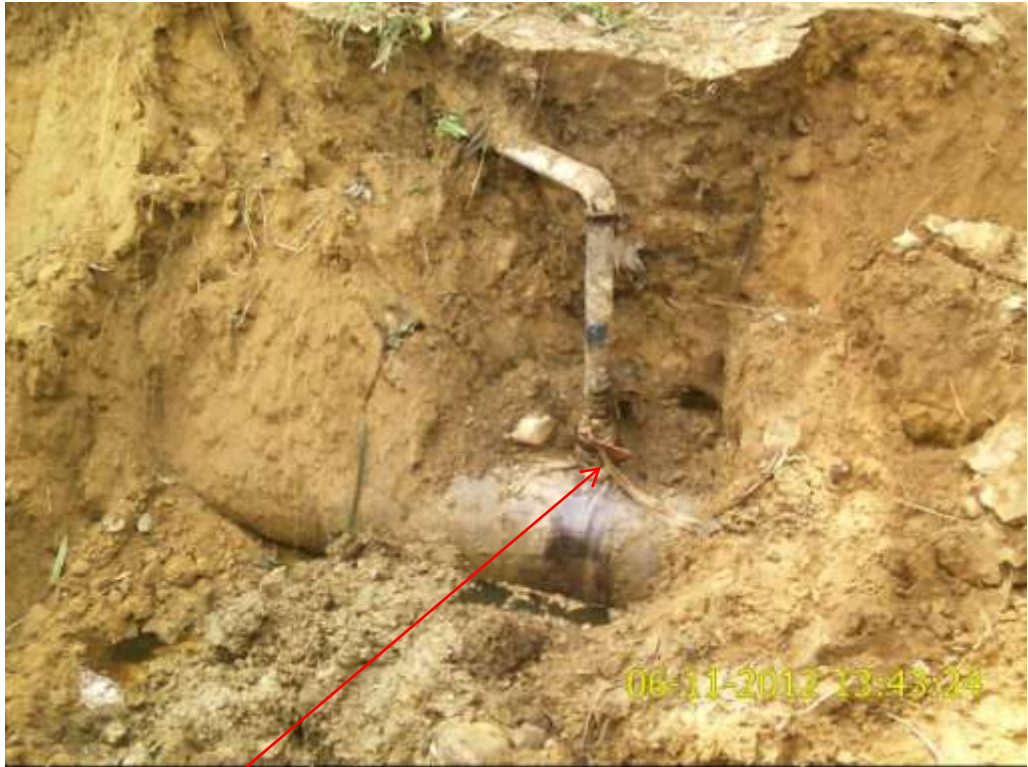
Close up: Illegal fitting on 24" Ogale-Bonny pipeline at Kpite. Picture was taken during Joint Investigation of 6 th November 2012.
