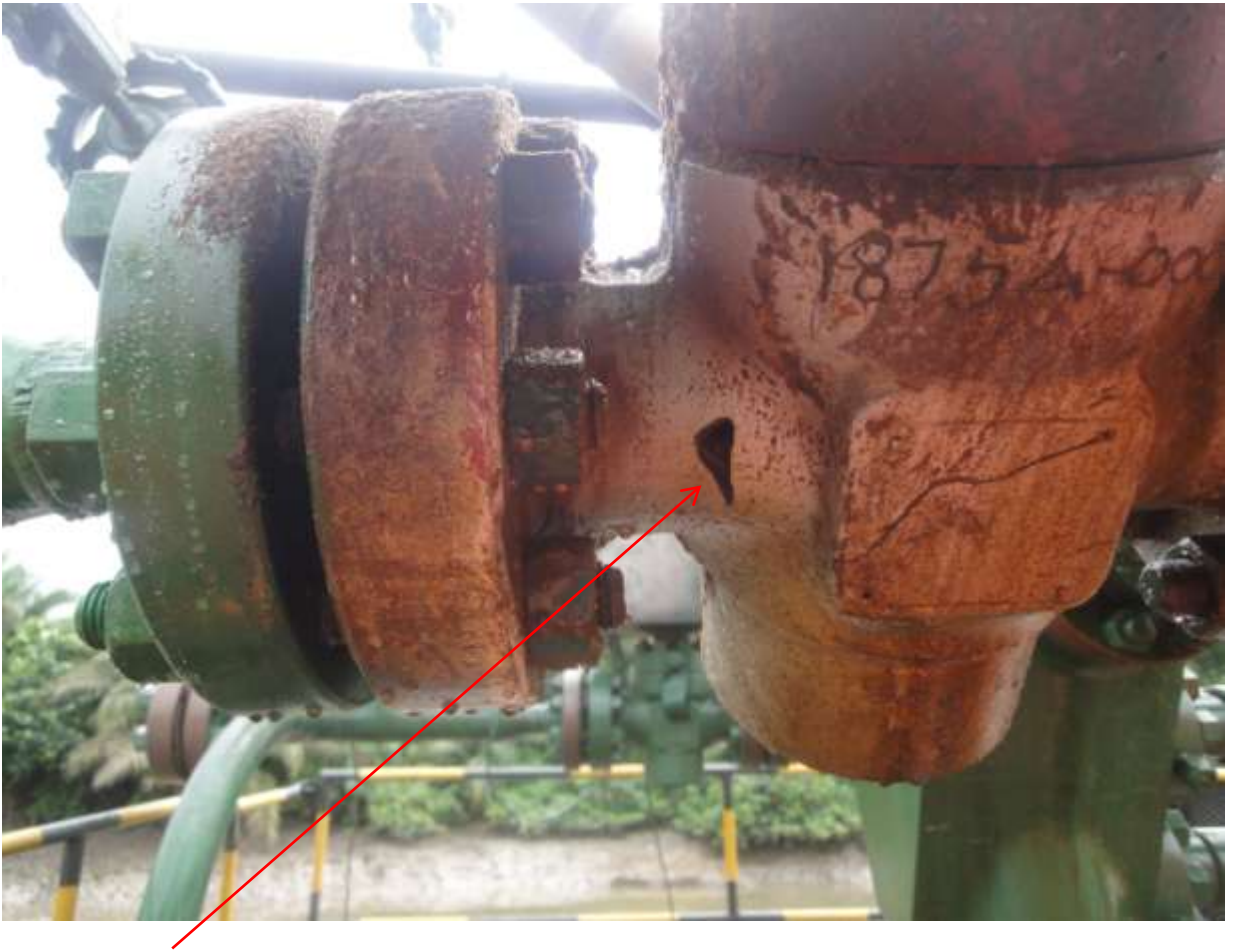
Close-up: Position of internal erosion on Nembe 1 Well 19S Wellhead at Ogbolomabiri. Picture was taken during Joint Investigation of 3 rd Dec. 2012.
