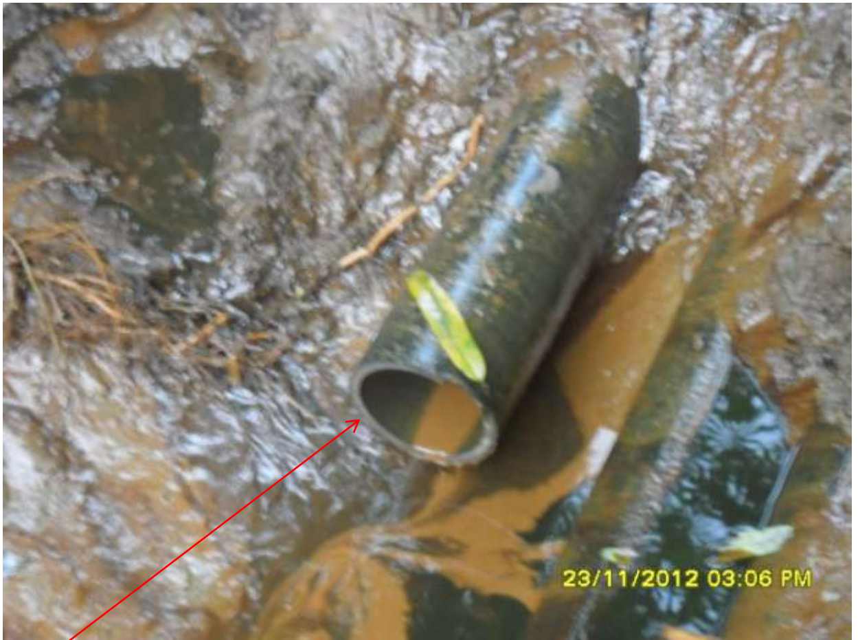
Close-up: Missing Flowline on Imo River Well 64S/L Flowline at Owaza. Picture was taken during Joint Investigation of 23 rd Nov. 2012.
