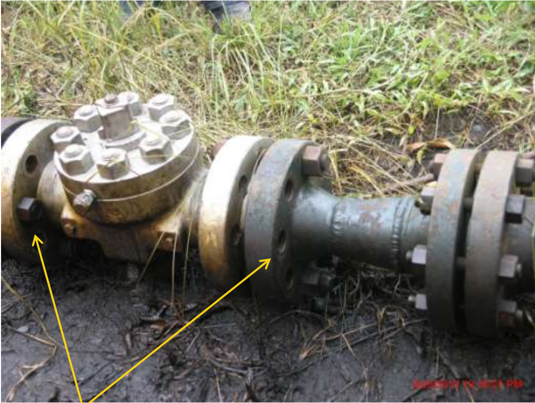
Close up: Missing bolts on Imo River2 Well28L flowline at Umuedeokwara. Picture was taken during Joint Investigation of 26 th May 2012.
