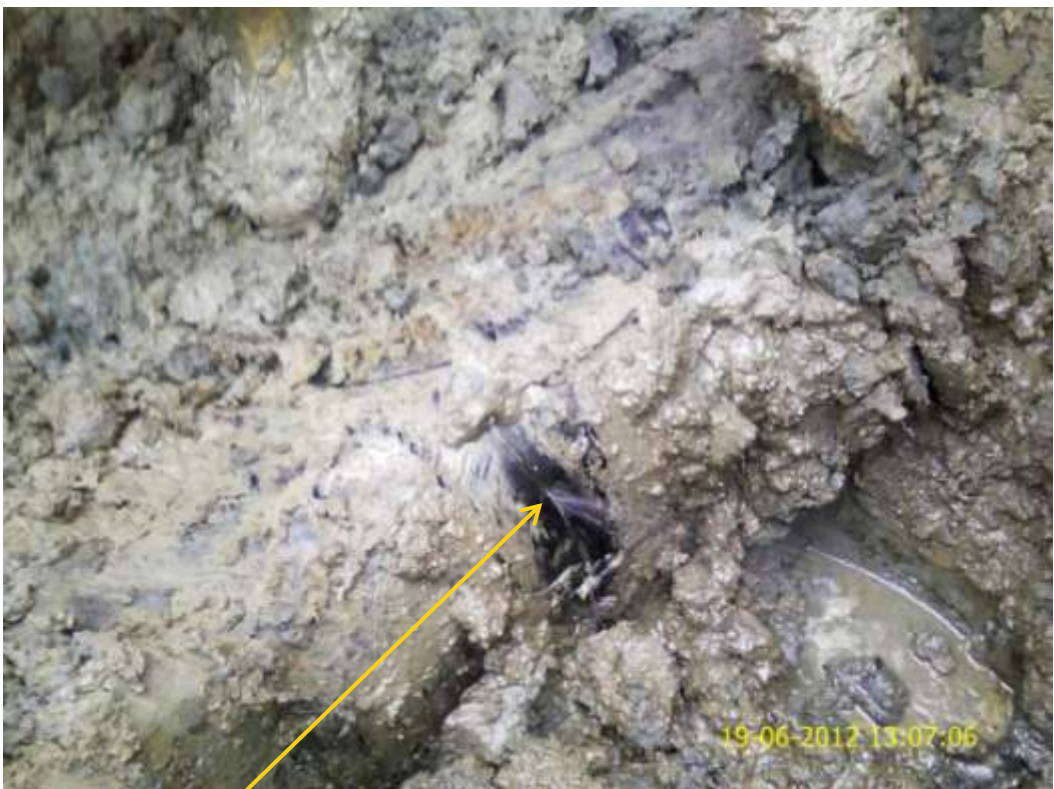
Close up: Hacksaw cut on 14" Okordia-Rumuekpe pipeline at Ikarama. Picture was taken during Joint Investigation of 19 th June 2012.
