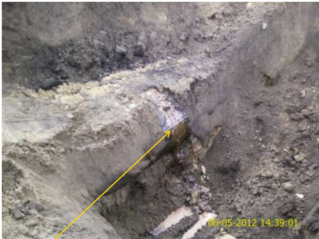
Close up: Hacksaw cut on 24" Bomu-Bonny pipeline at Mogho. Picture was taken during Joint Investigation of 6 th May 2012.
