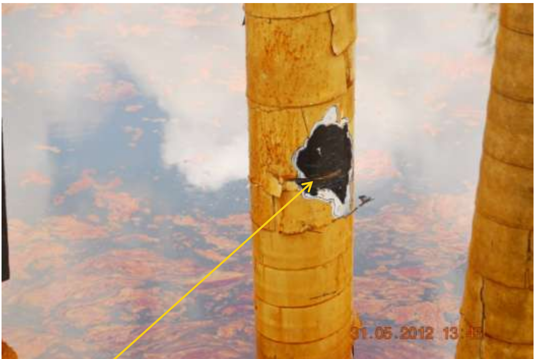
Close up: Hacksaw cut on Benisede Well 1 flowline at Tamogbene. Picture was taken during Joint Investigation of 31 st May 2012.
