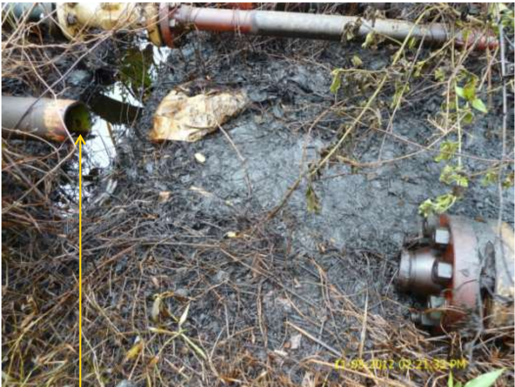
Close up: Cut section on 4" Agbada2 Well48S flowline at Omuohia . Picture was taken during Joint Investigation of 11 th May 2012.
