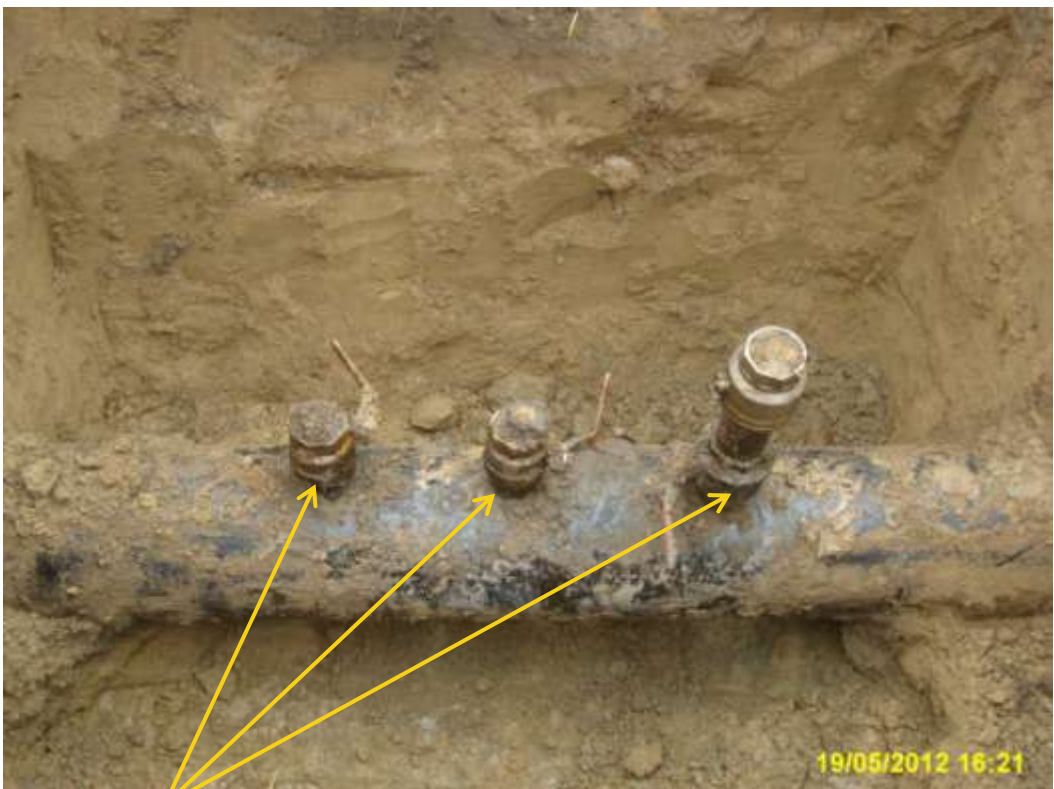
Close up: Illegal fittings on 12" Imo River1 pipeline at Uzuaku. Picture was taken during Joint Investigation of 19 th May 2012.
