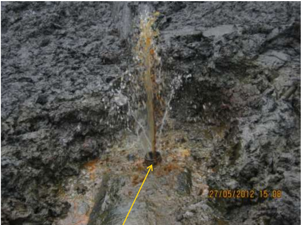
Close up: Illegal fitting on 24" Nembe Creek Trunkline behind Sego Manifold. Picture was taken during Joint Investigation of 27 th May 2012.
