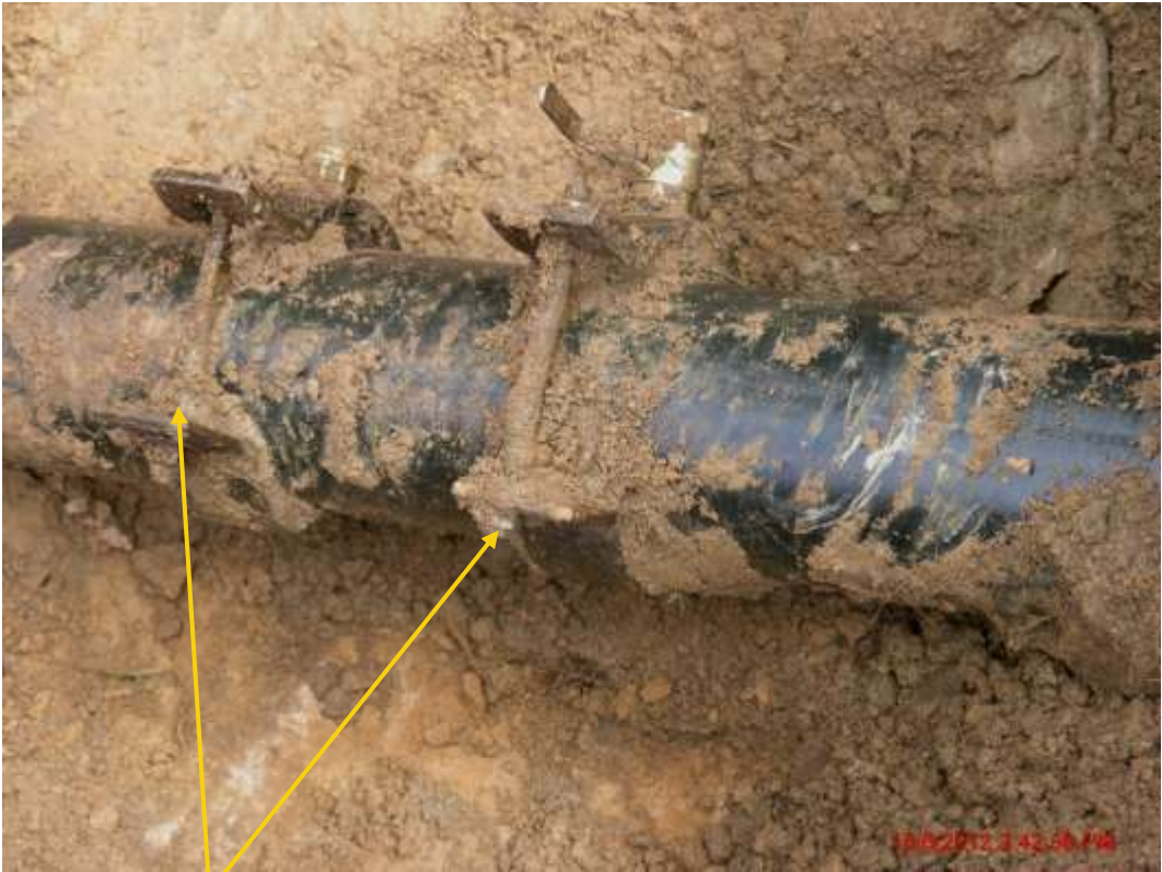
Close up: Illegal fittings on Imo River1 Well59T flowline at Igiriukwu. Picture was taken during Joint Investigation of 15 th June 2012.
