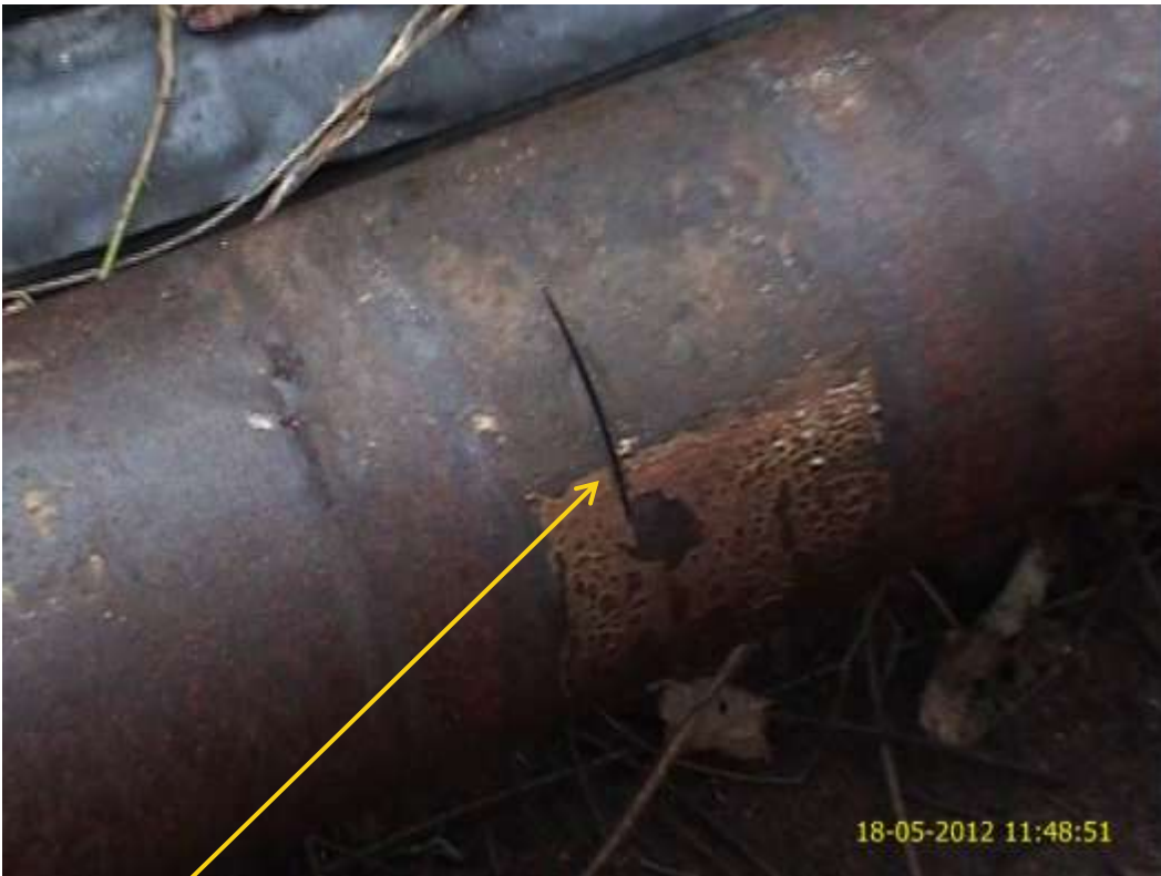
Close up: Hacksaw cut on Imo River1 Well26L flowline at Owaza. Picture was taken during Joint Investigation of 5 th May 2012.
