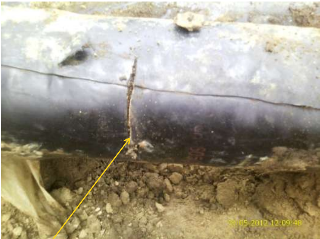
Close up: Hacksaw cut on Agbada Well34S flowline at Omuohia Omueke. Picture was taken during Joint Investigation of 31 st May 2012.
