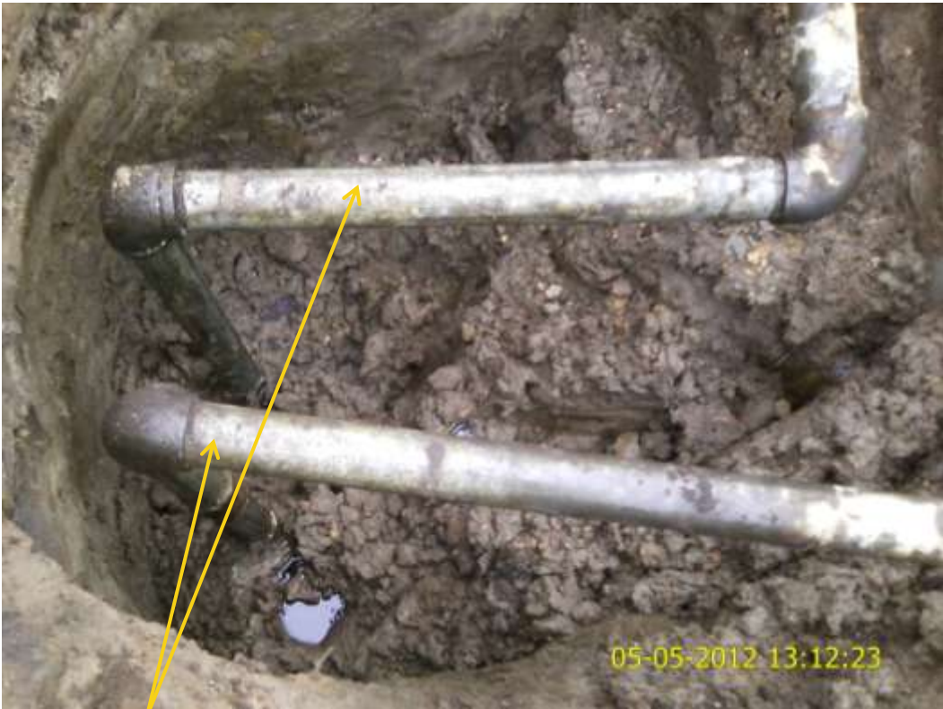
Close up: Illegal fittings on 12" Imo River2 pipeline at Odagwa. Picture was taken during Joint Investigation of 5 th May 2012.
