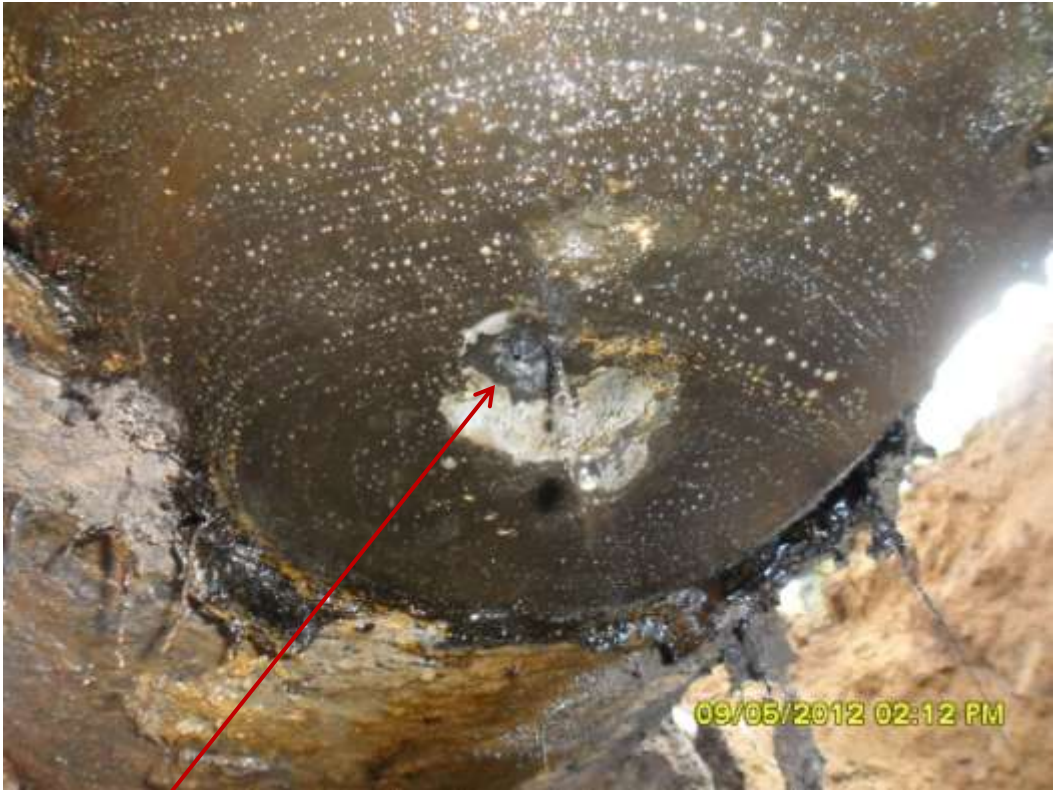
Close up: Leak point, due to corrosion, at 6 o' clock position on 28" Bomu-Bonny pipeline at K-Dere. Picture was taken during Joint Investigation of 9 th May 2012.
