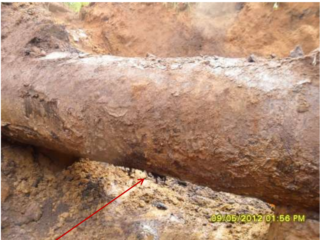
Close up: Leak point, due to corrosion, at 6 o' clock position on 28" Bomu-Bonny pipeline at K-Dere. Picture was taken during Joint Investigation of 9 th May 2012.
