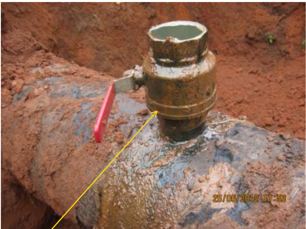
Close up: Illegal fitting on 16" Egbema-Assa trunkline at Obile. Picture was taken during Joint Investigation of 26 th May 2012.
