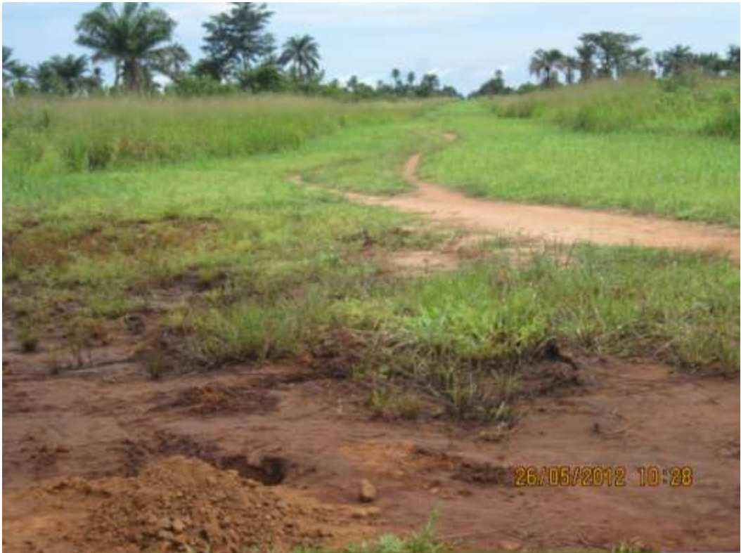
Overview: Part of spill impact on 16" Egbema-Assa trunkline right of way at Obile. Picture was taken during Joint Investigation of 26 th May 2012.
