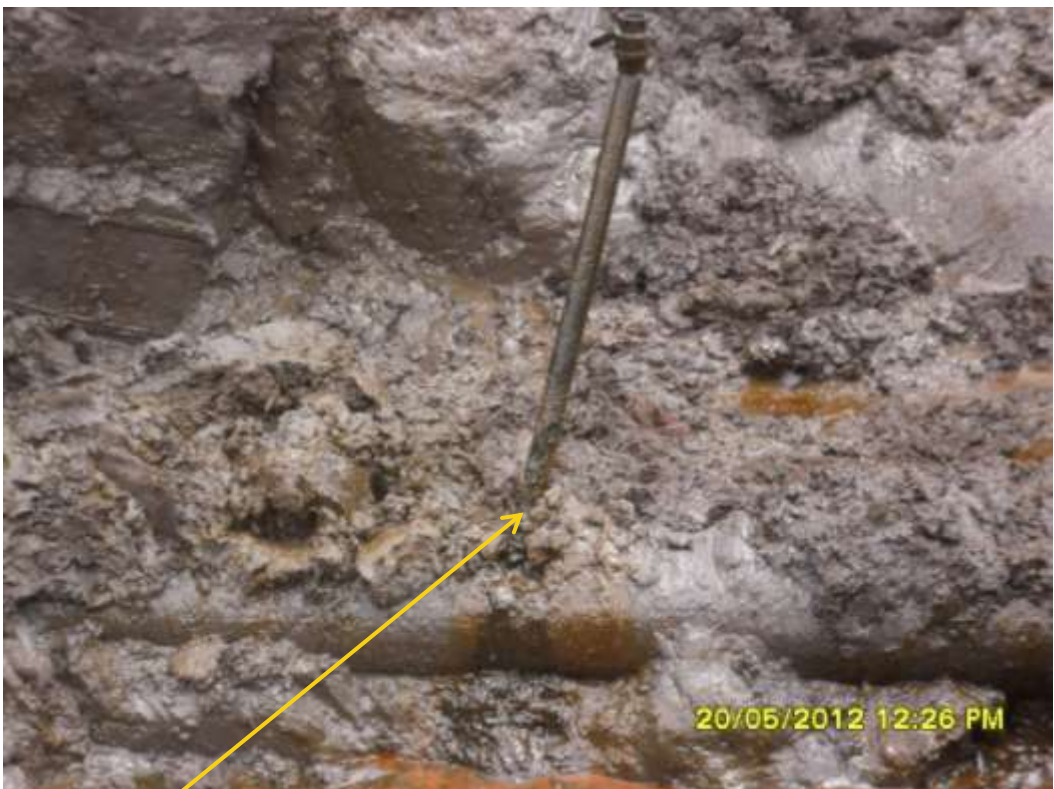
Close up: Illegal fitting on 10" Ekulama1-Sanbarth pipeline at Ekulama1. Picture was taken during Joint Investigation of 20 th May 2012.
