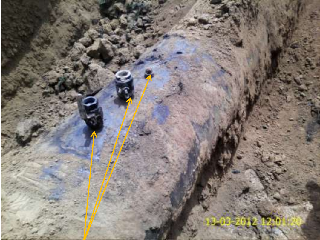
Close up: Illegal fittings on 36" Rumuekpe-Nkpoku pipeline at Mbodo-Aluu. Picture was taken during Joint Investigation of 13 th March 2012.
