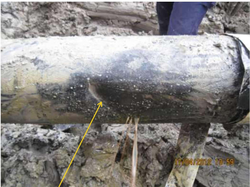
Close up: Inward dent on 10" Diebu Creek – Nun River pipeline at Oporoma. Picture was taken during Joint Investigation of 17 th April 2012.
