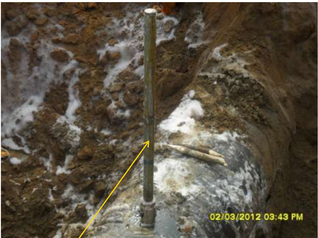
Close up: Illegal fitting on 36" Rumuekpe-Nkpoku pipeline at Omuigwe-Aluu. Picture was taken during Joint Investigation of 2 nd March 2011.
