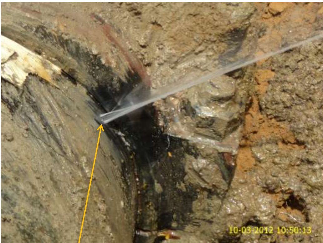
Close up: Hacksaw cut on 24" Nkpoku-Bomu pipeline at Egballor. Picture was taken during Joint Investigation of 10 th March 2012.
