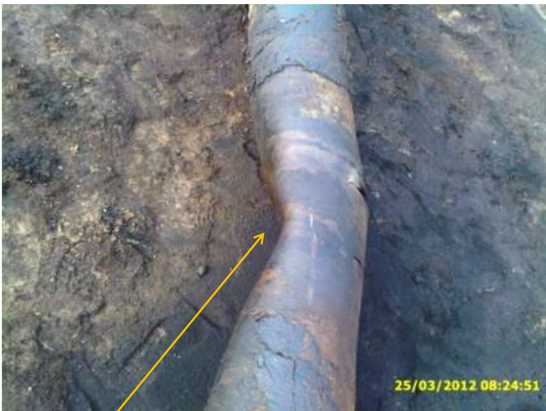
Close up: Inward dent and tear on 12" Kokori-Eriemu delivery line at Oteri. Picture taken during repair of delivery line on 25 th March 2012.
