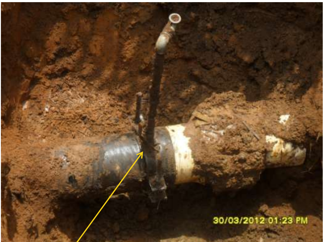
Close up: Illegal fitting on 8" Umuechem-Nkpoku pipeline at Umuechem. Picture was taken during Joint Investigation of 30 th March 2012.
