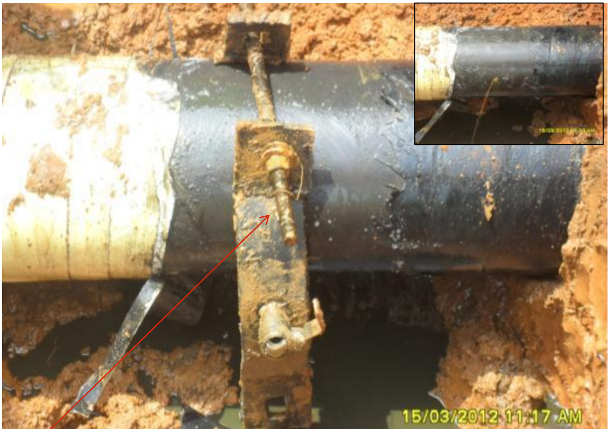
Close-up: Illegal fitting on 8" Nkali pipeline at Odagwa. Picture was taken during Joint Investigation of 15 th March, 2012.
