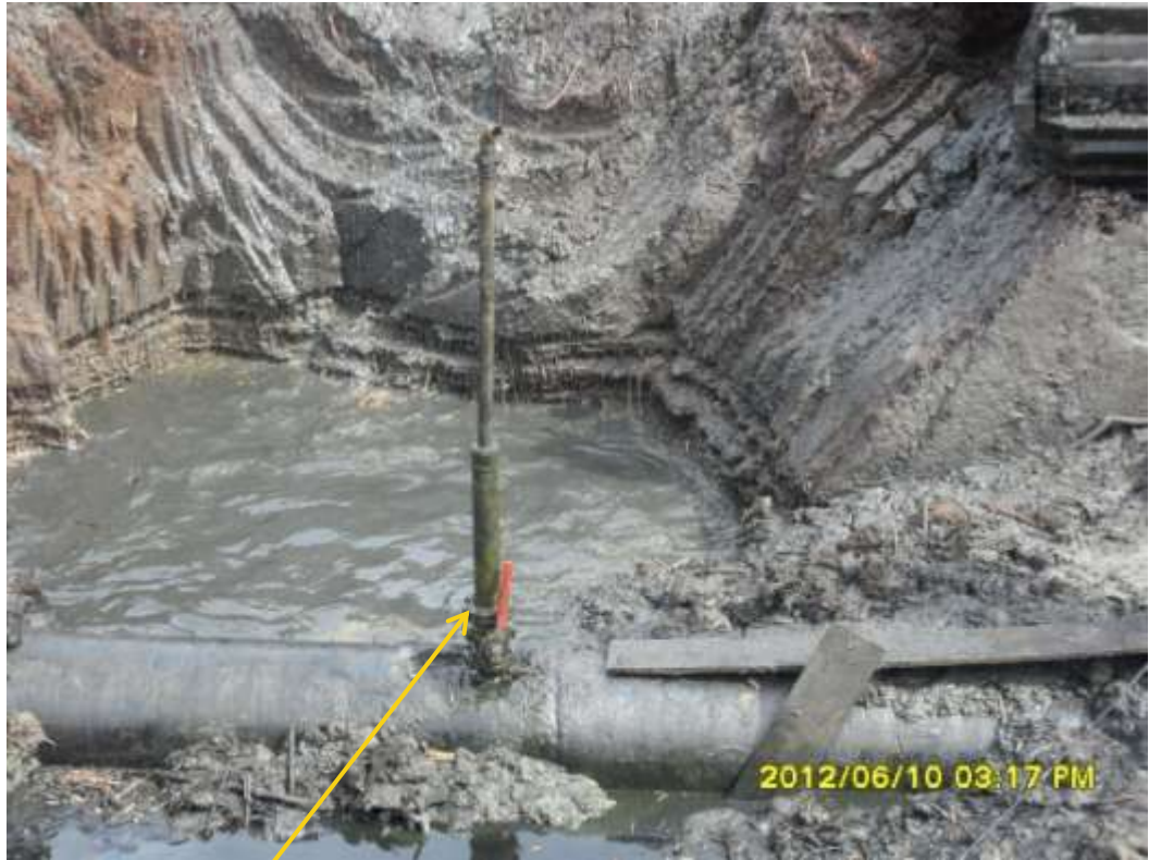
Close up: Illegal fitting on 24" Nembe Creek pipeline at Segoo. Picture was taken during Joint Investigation of 10 th June 2012.
