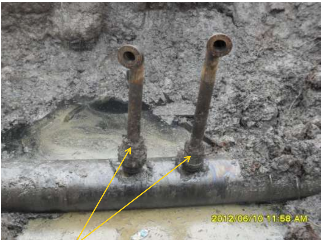
Close up: Illegal fittings on 24" Nembe Creek pipeline at Segoo. Picture was taken during Joint Investigation of 10 th June 2012.
