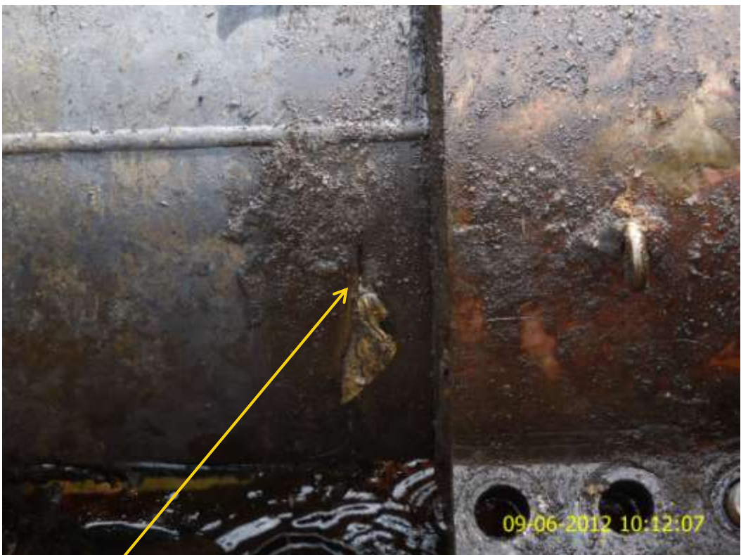
Close up: Hacksaw cut on 24" Npoku-Bomu pipeline at Bera. Picture was taken during Joint Investigation of 9 th June 2012.
