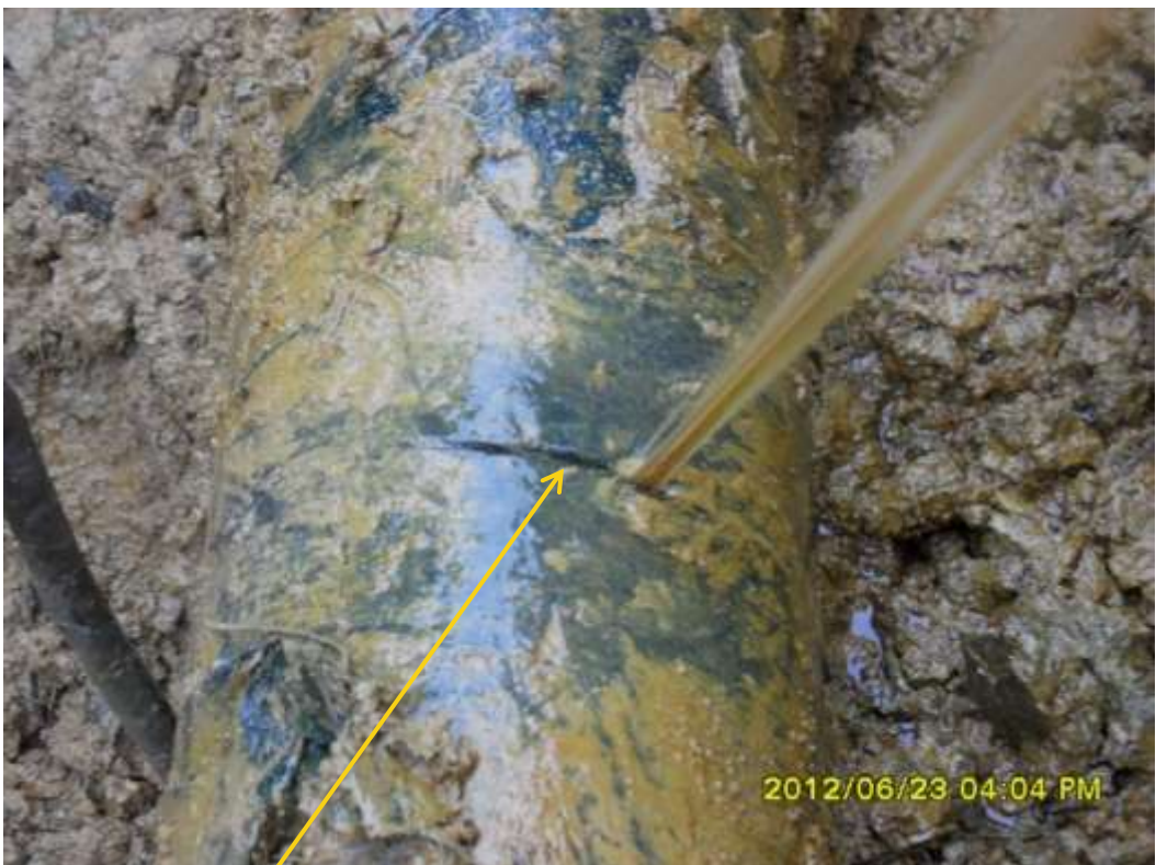
Close up: Hacksaw cut on 10" Diebu Creek pipeline at Onyoma. Picture was taken during Joint Investigation of 23 rd June 2012.
