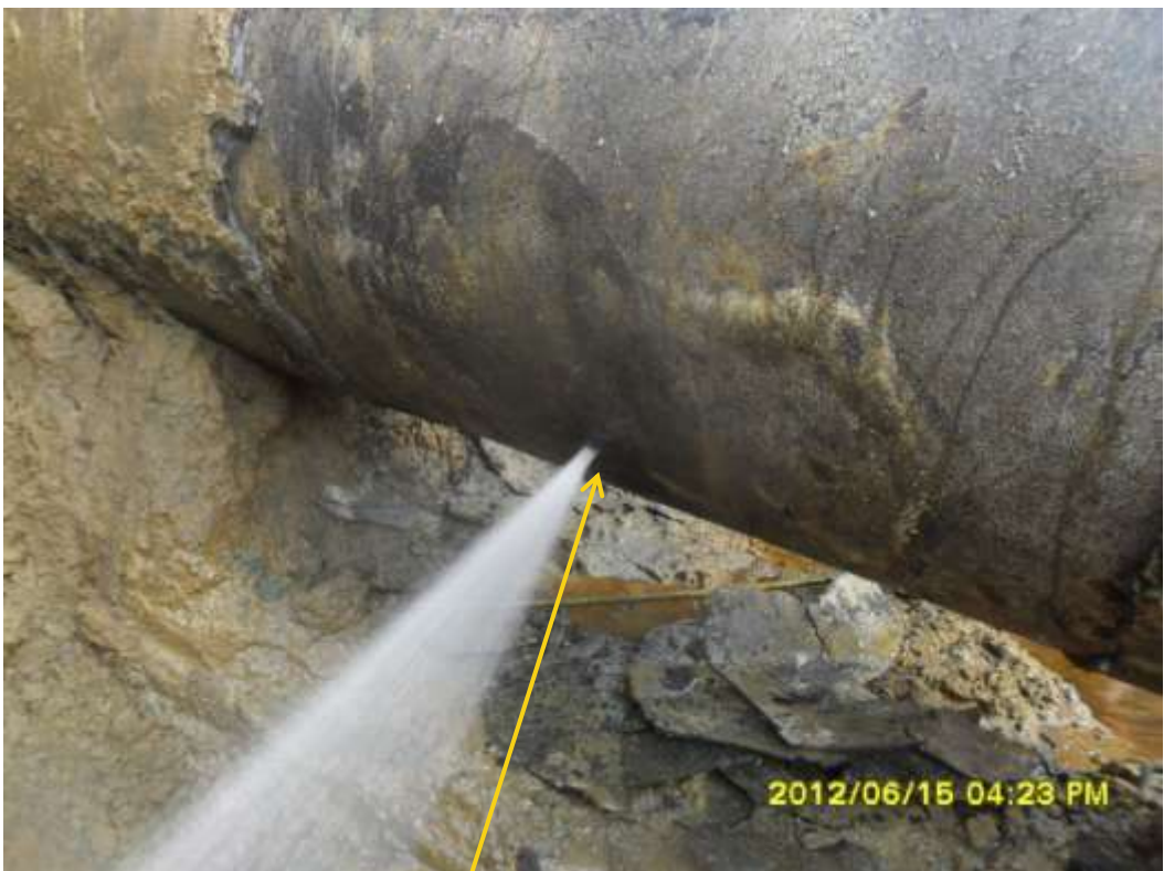
Close up: Spill point due to corrosion on 24" Npoku-Bomu pipeline at Ogale. Picture was taken during Joint Investigation of 15 th June 2012.
