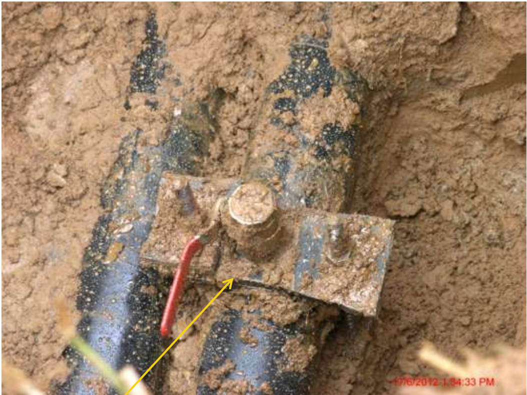
Close up: Illegal fitting on Agbada2 Well69S flowline at Umuokwa. Picture was taken during Joint Investigation of 17 th June 2012.
