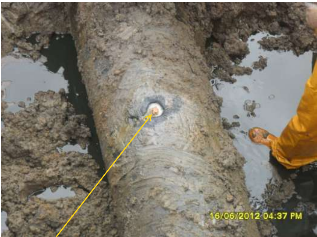
Close up: Drilled hole on 20" Rumuekpe-Nkpoku trunkline at Ibaa. Picture was taken during Joint Investigation of 16 th June 2012.
