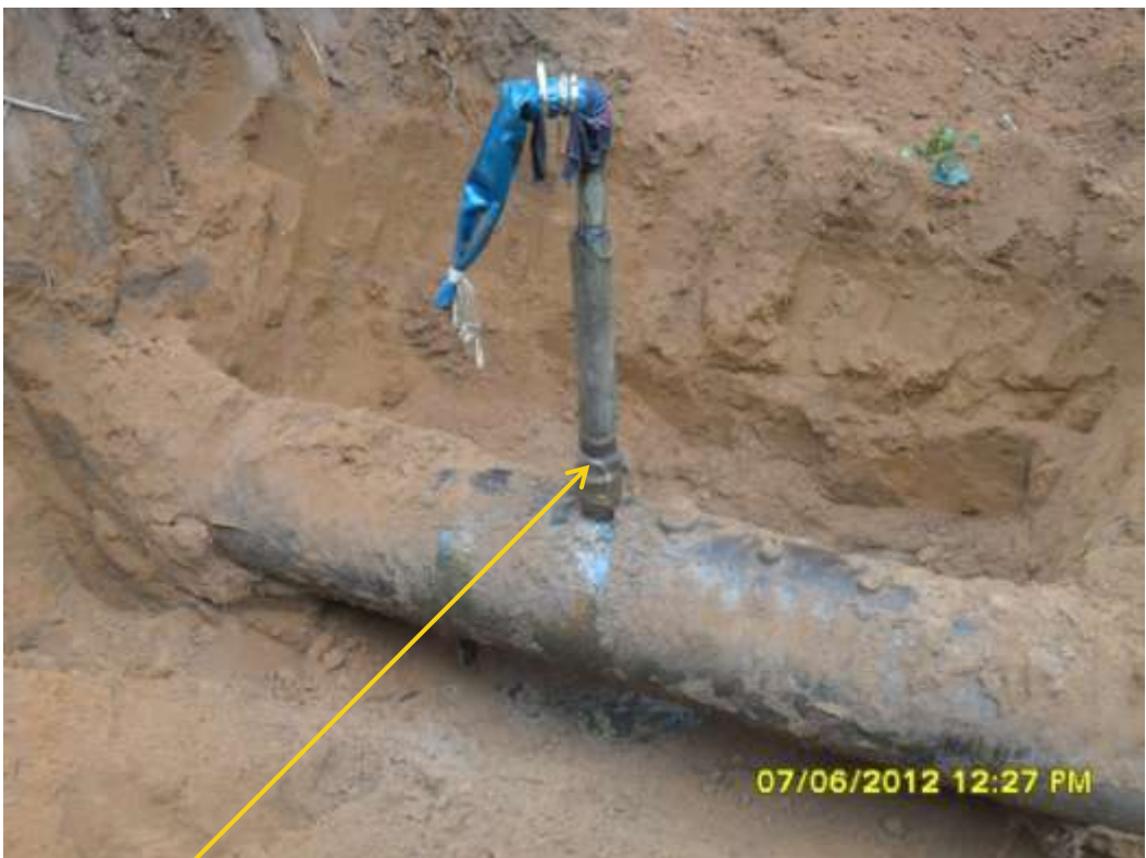
Close up: Illegal fitting on 18" Assa-Rumuekpe pipeline at Omudioga. Picture was taken during Joint Investigation of 7 th June 2012.
