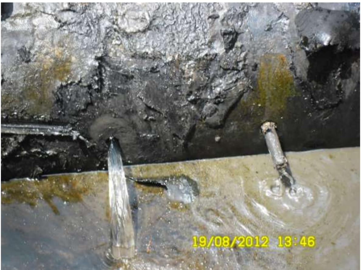
Close-up: Drilled holes on 24" Alakiri – Bonny Pipeline at Kalibiama. Picture was taken during Joint Investigation of 19 th August 2012.
