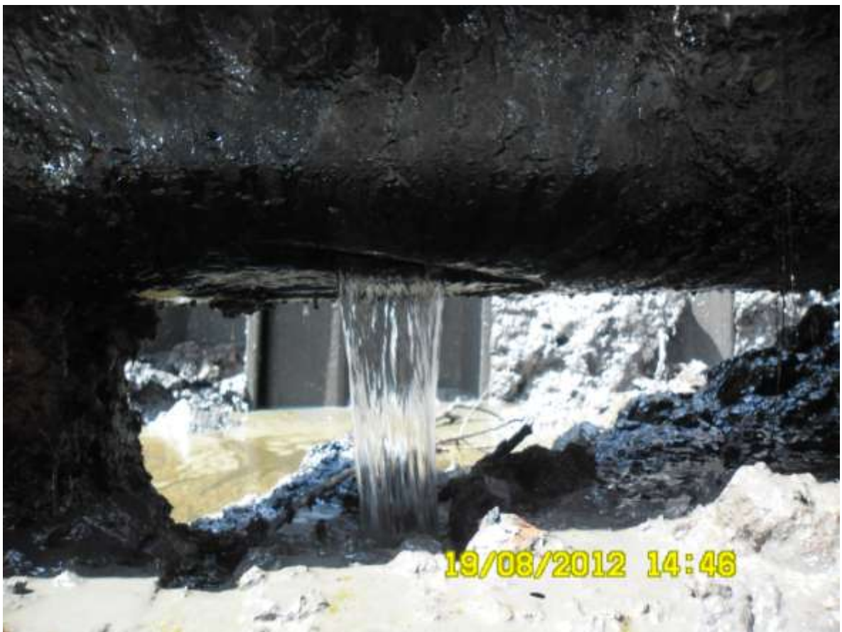
Close-up: External grind off surface on 24" Alakiri – Bonny Pipeline at Kalibama. Picture was taken during Joint Investigation of 19 th August 2012
