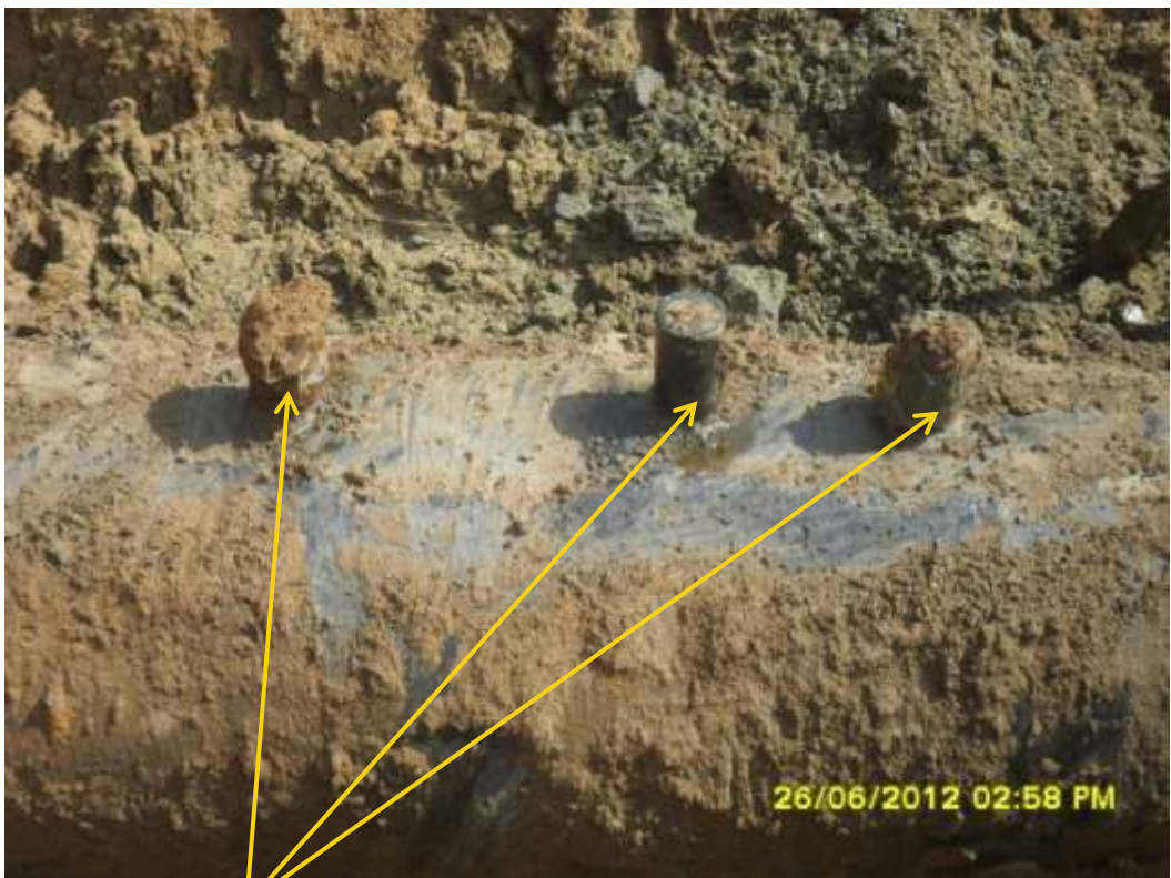
Close up: Illegal fittings on 24" Npoku-Bomu trunkline at Botem. Picture was taken during Joint Investigation of 26 th June 2012.
