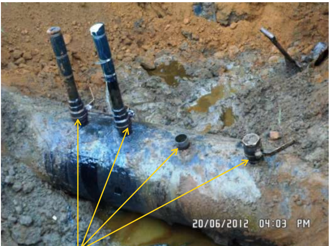
Close up: Illegal fittings on 24" Npoku-Bomu Trans Niger Pipeline at Nonwa. Picture was taken during Joint Investigation of 20 th June 2012.
