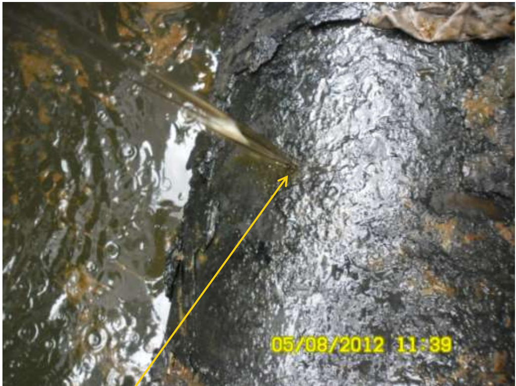
Close up: Pinhole leak on 24" Alakiri-Bonny pipeline at Fusokiri/Ilomaturu located through injection of pressure on the line on 2 nd August 2012. Picture was taken during Joint Investigation of 5 th August 2012.
