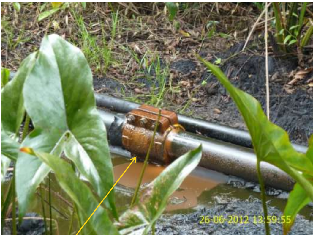
Close up: Failed clamp on Imo River Well5 flowline at Igrukwu. Picture was taken during Joint Investigation of 26 th June 2012.
