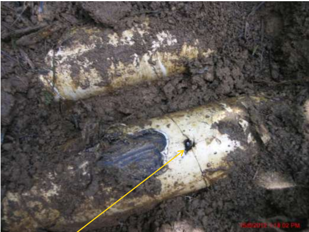
Close up: Drilled hole on Obigbo North Well28LS flowline at Imeh. Picture was taken during Joint Investigation of 15 th June 2012.
