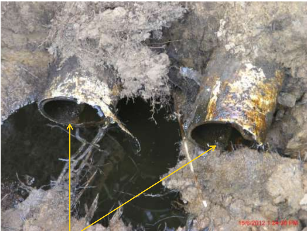
Close up: Cut flowline sections on Obigbo North Well28LS flowline at Imeh. Picture was taken during Joint Investigation of 15 th June 2012.
