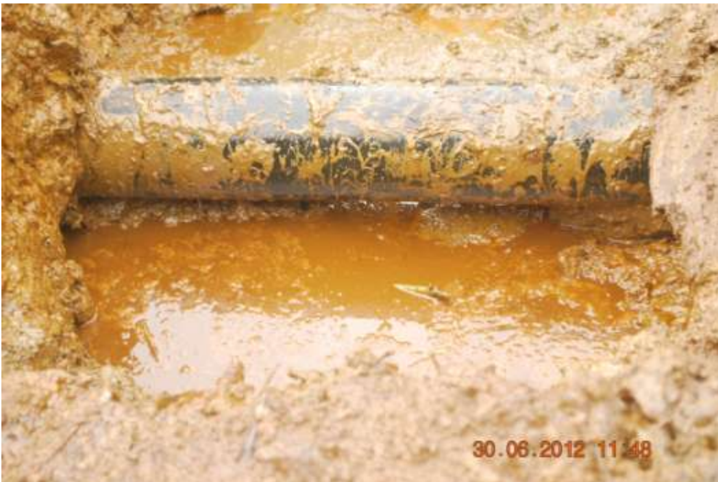
Close up: Spill due to corrosion on Opukushi Well24T flowline at Agbemo-Angalebiri. Picture was taken during Joint Investigation of 30 th June 2012.
