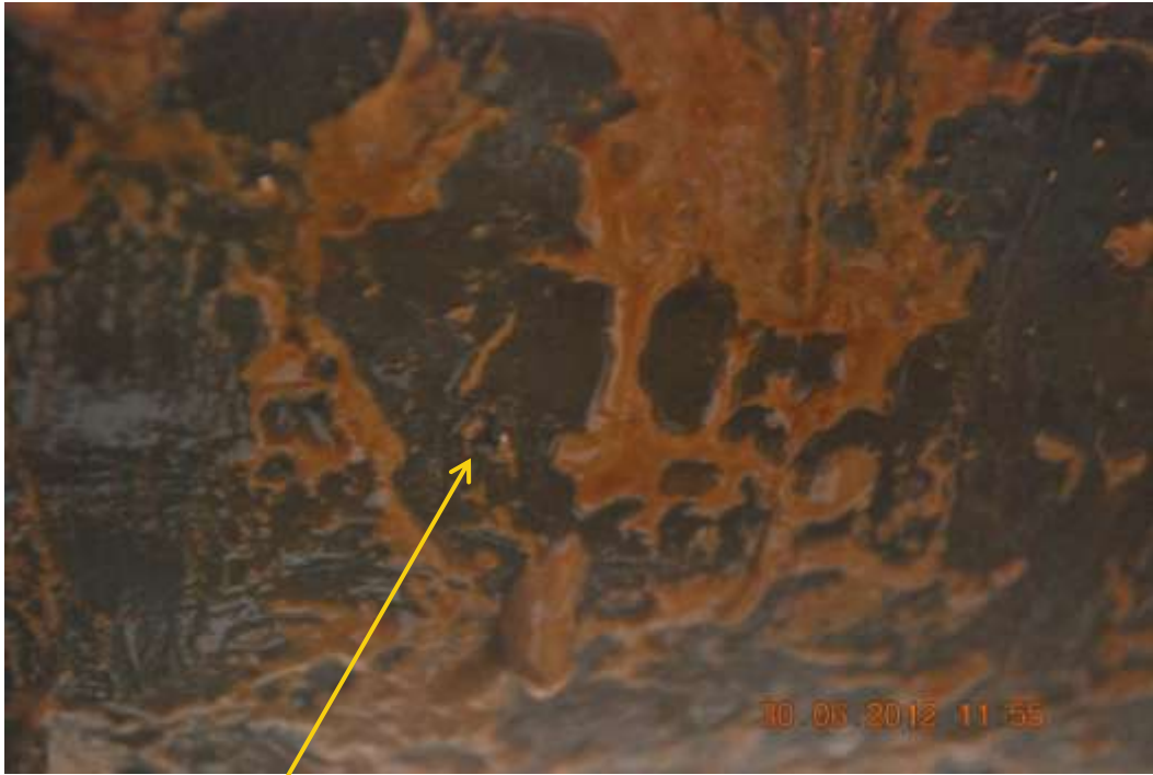
Close up: Spill due to corrosion at 6 o'clock position on Opukushi Well24T flowline at Agbemo-Angalebiri.
