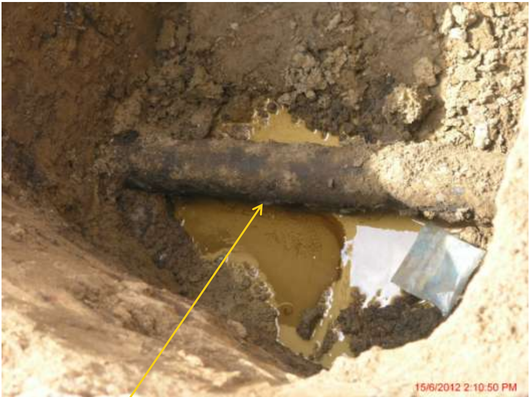
Close up: Spill due to corrosion on Obigbo North Well03L flowline at Umuebulu. Picture was taken during Joint Investigation of 15 th June 2012.
