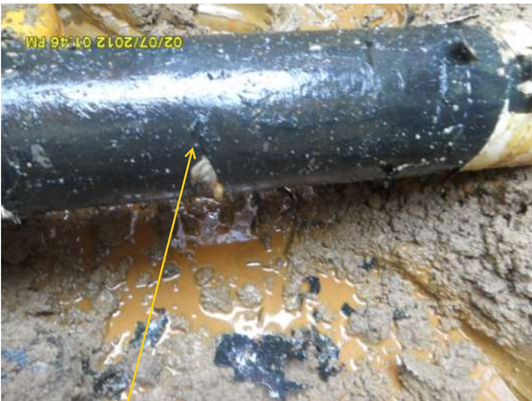
Close up: Spill due to Hacksaw cut on 4" Obele-Ibaa pipeline at Ibaa. Picture was taken during Joint Investigation of 2 nd July 2012. (Picture was rotated for clarity)
