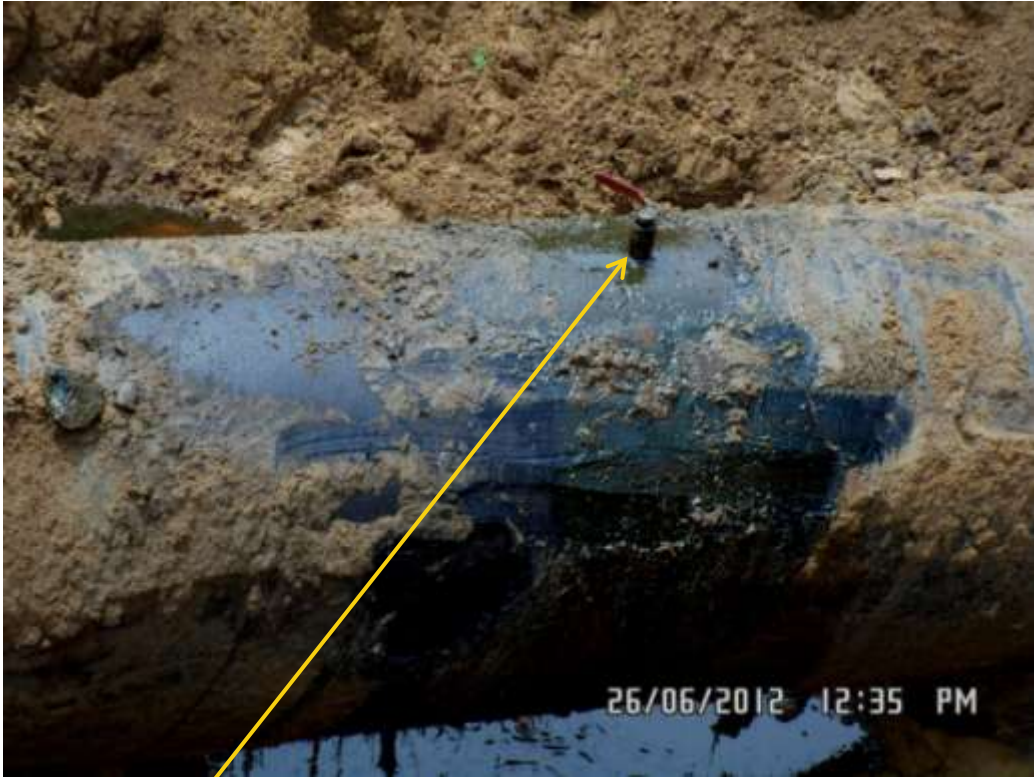
Close up: Illegal fitting on 28" Nkpoku-Bomu pipeline at Gio. Picture was taken during Joint Investigation of 26 th June 2012.
