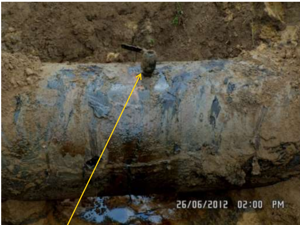
Close up: Illegal fitting on 28" Nkpoku-Bomu pipeline at Gio. Picture was taken during Joint Investigation of 26 th June 2012.
