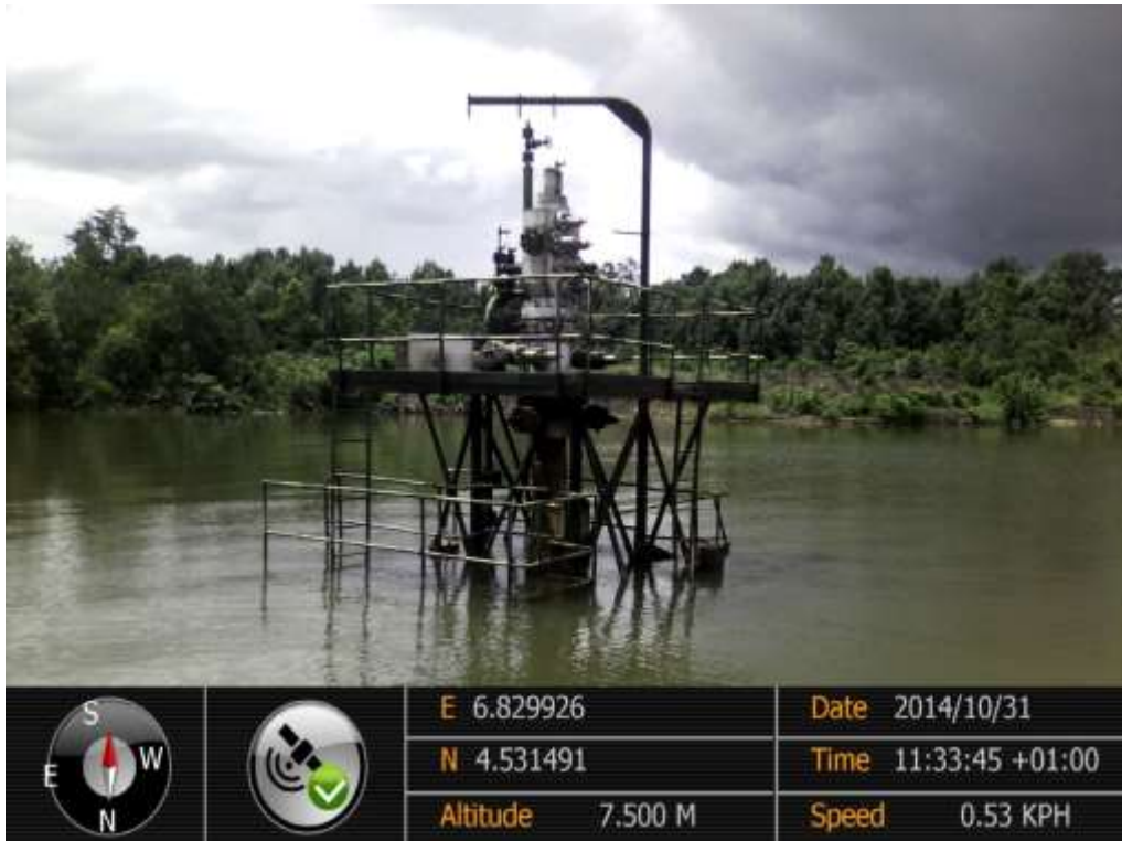
Overview: Site of spill on Awoba Well8T Flowline Right of Way at Bille. Picture was taken during Joint Investigation of 31 st October 2014.
