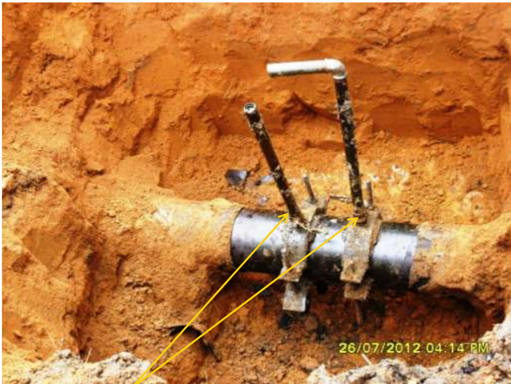
Close up: Illegal fittings on 8" Umuechem-Nkpoku pipeline at Omusele. Picture was taken during Joint Investigation of 26 th July 2012.
