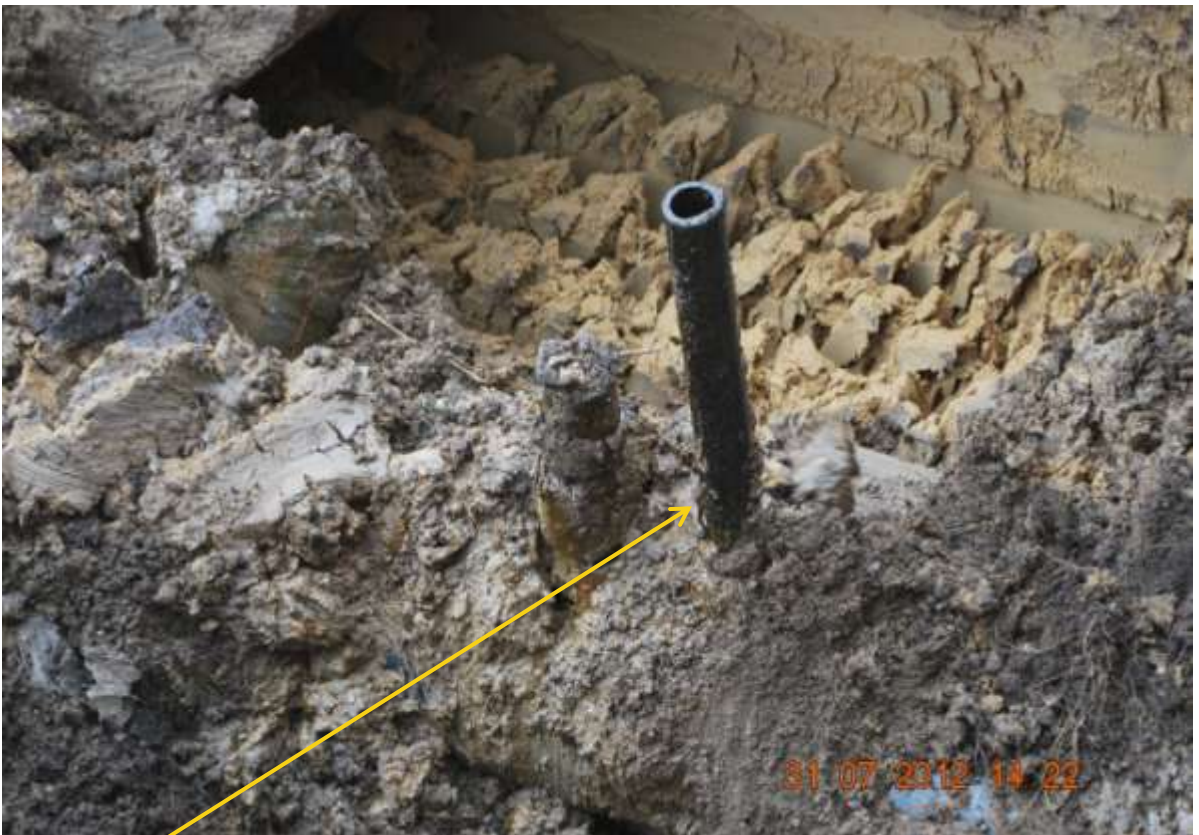
Close-up: Illegal fitting on 12" Afiesere - Eriemu Delivery Line at Emeragha. Picture was taken during Joint Investigation of 31 st July, 2012
