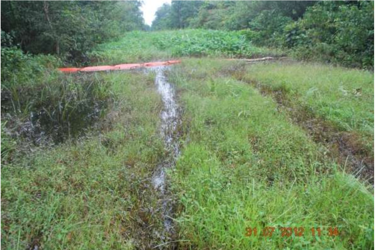
Overview: Part of spill impact on 12" Afiesere - Eriemu Delivery Line at Emeragha. Picture was taken during Joint Investigation of 31 st July, 2012.
