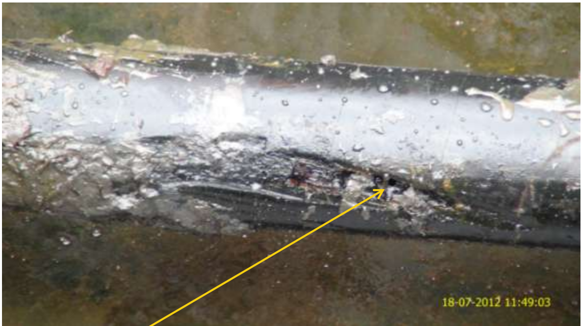
Closeup: Pinhole on Cawthorne Channel 2 Well51T flowline at Mbiama. Picture was taken during Joint Investigation of 18 th July 2012.
