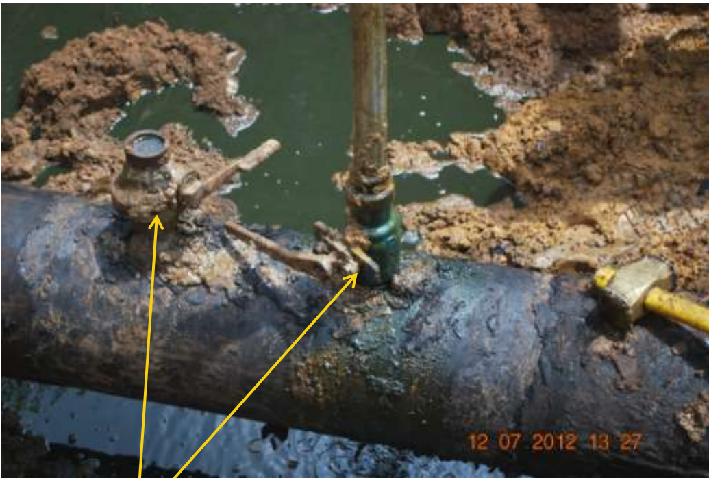
Close up: Illegal fittings on 12" Kokori-Eriemu pipeline at Omavovwe. Picture was taken during Joint Investigation of 12 th July 2012.
