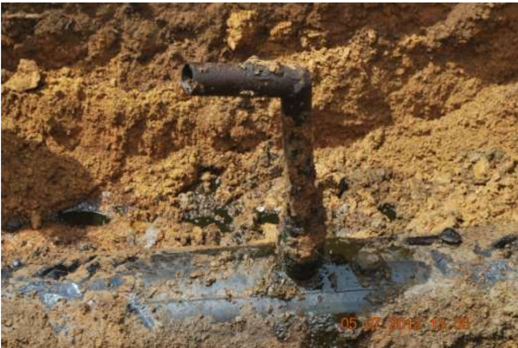
Close up: Illegal fitting on 16" Uzere-Eriemu trunkline at Iyede. Picture was taken during Joint Investigation of 5 th July 2012.
