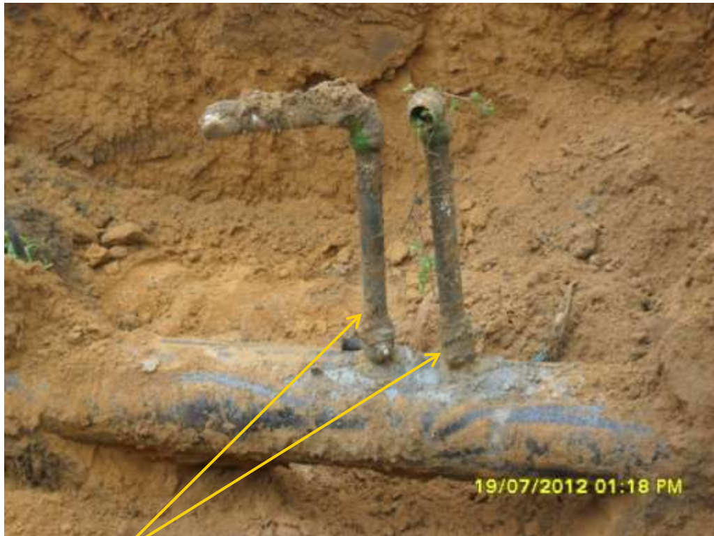
Close up: Illegal fittings on 12" Imo River2 – Ogale pipeline at Owaza. Picture was taken during Joint Investigation of 19 th July 2012.
