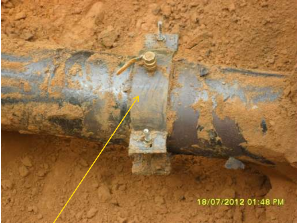
Close up: Illegal fitting on 12" Imo River2 – Ogale pipeline at Owaza. Picture was taken during Joint Investigation of 18 th July 2012.
