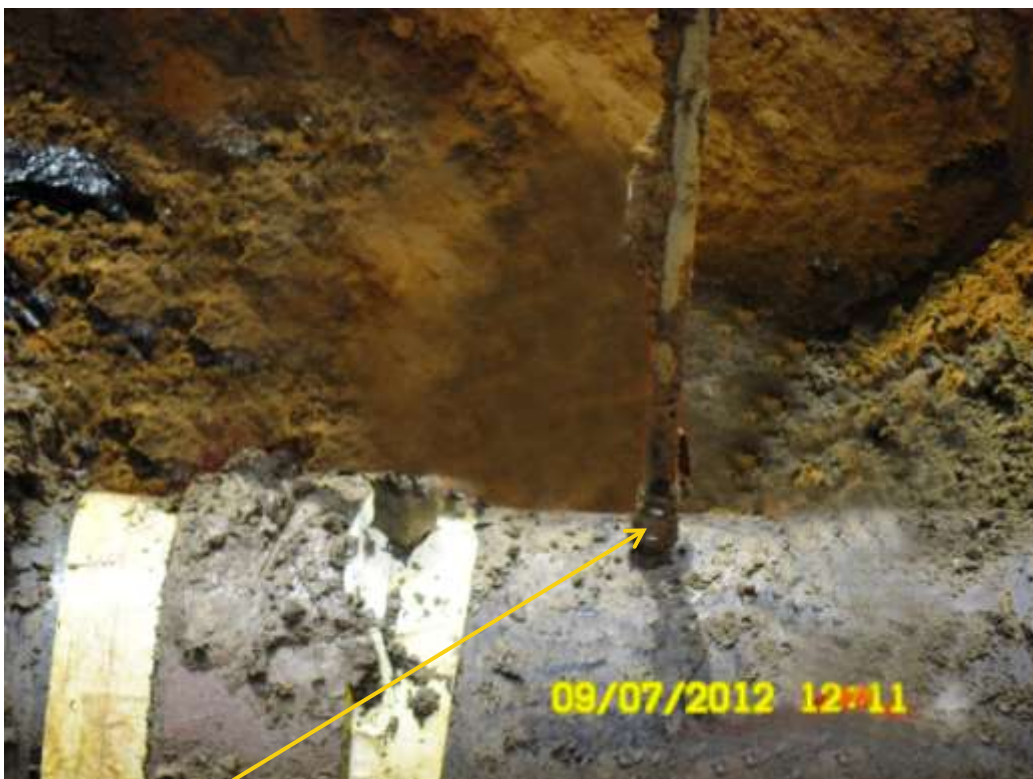
Close up: Illegal fitting on 36" Rumuekpe-Nkpoku Trans Niger Pipeline at Mgbodo-Aluu. Picture was taken during Joint Investigation of 9 th July 2012.
