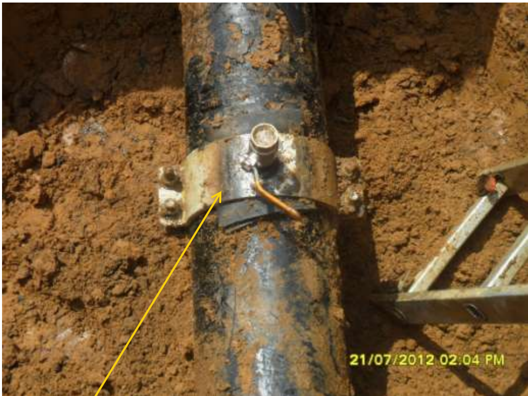
Close up: Illegal fitting on 8" Umuechem-Nkpoku delivery line at Umuechem. Picture was taken during Joint Investigation of 21 st July 2012.
